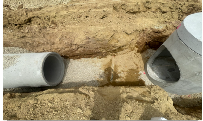
Picture of water main conflict with storm off windmill ridge
